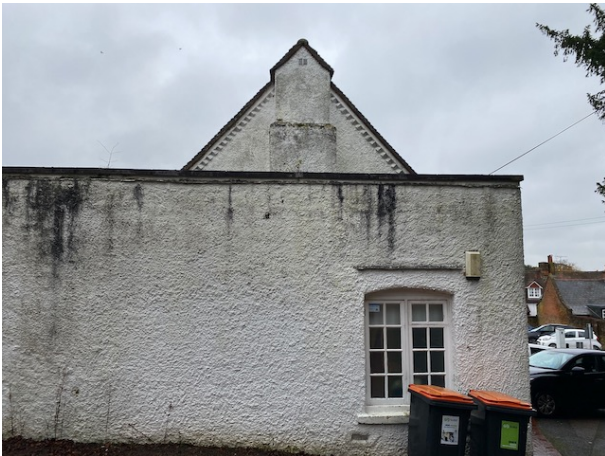
Parapet to MP's office: Detailing to shed water is poor, potentially resulting in moisture entering the top of the wall. No access into roof void over, with potential risk of decay
