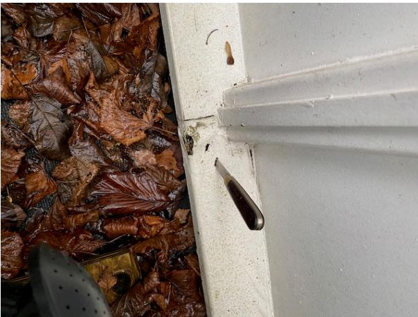
Areas of timber decay in external joinery
