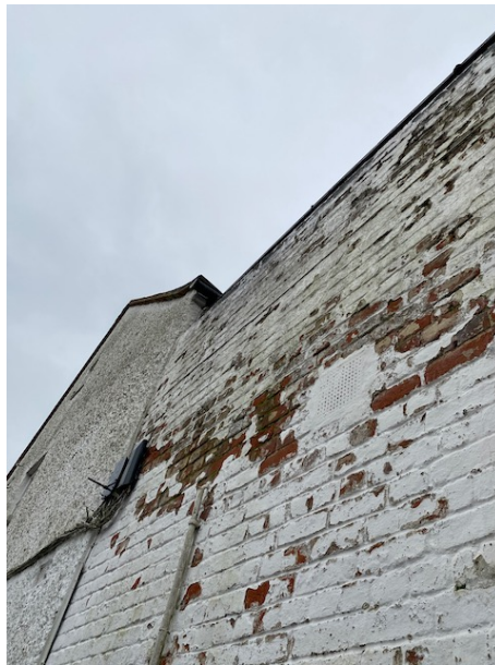
North wall of link. Internal surface of wall corresponding to problems noted externally
