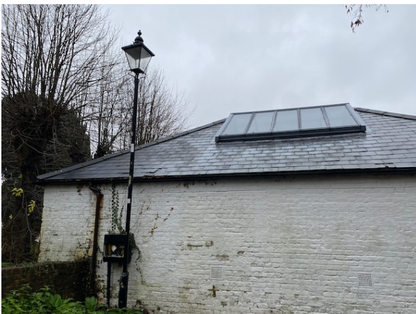
Roof to Library: Slates damaged around lamp post and along line of eaves (attempted break in?)
