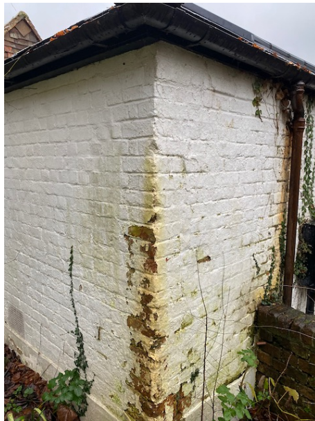
Damp running over walls causing paint to fail and risking dry rot inside the building
