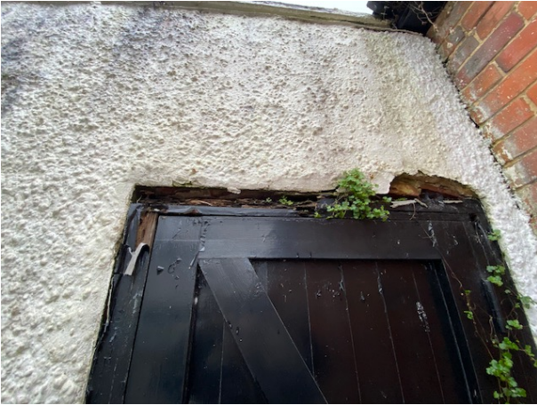
Timber frame to door failed, potentially compromising support over
