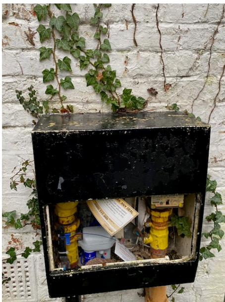
Damage to gas meter housing: URGENT
