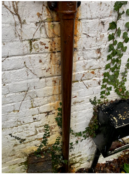
Blocked and rusting gutters and downpipes saturating the wall behind
