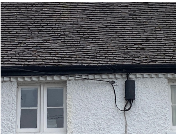
Front elevation roof: Slight sag in line of roof over window. Slipped and missing tiles
